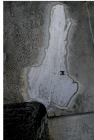
Fig. 9: Locations of hardness measurement in the area III (crack vicinity).
