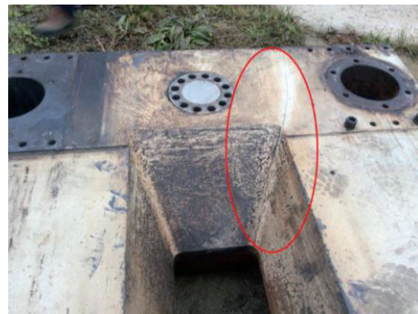
Fig. 6: Fixed plate with crack.
