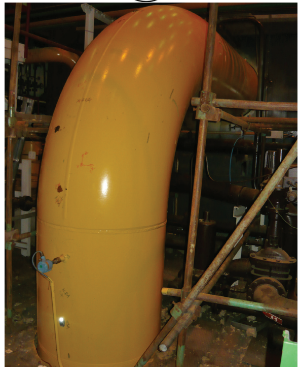
Fig. 1: Output pipe of turbocompressor. a) scheme of pipe, b) view at output pipe above terrain level (ground).
